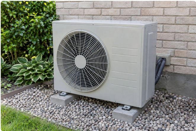
AC-02 after service • External panels closed and surrounding area clear.
